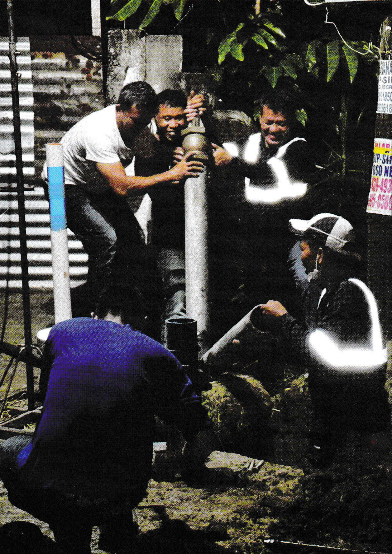
PRIMEWATER PERSONNEL GEORGE R. BARLONGAY, ENRICO JANABAN, NOEL M. MARANO, SERGIO F. FORTES AND JONNEL JIMENA INSTALLING AN ADDITIONAL FIRE HYDRANT AT PHASE III LAST JUNE 10 IN PREPARATION FOR OPLAN LINIS TUBO ACTIVITIES NEXT MONTH.
