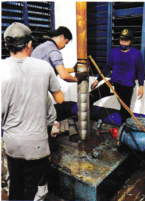
PrimeWater plumbers installing a new submersible pump and motor for Baribag Pumping Station, Apr. 26
