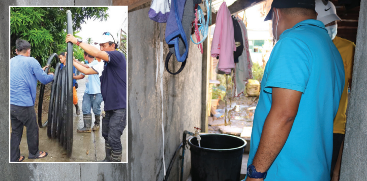
IGM Engr. Eduardo P. Tejada checks the water supply at Janaban residence, Miraculous Subdivision, Brgy. Macabog on Feb. 26, weeks after PrimeWater plumbers (inset) installed an additional 2-in diameter distribution line on Feb. 8.
